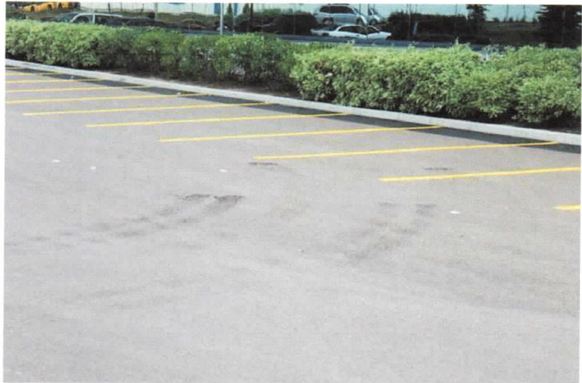
Typical view of tire marking in a pavement constructed to meet all OPSS standards but opened to truck traffic within 6 hours of paving.
