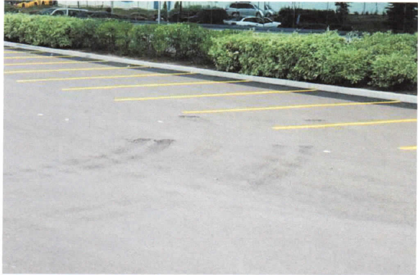
Typical view of tire marking in a pavement constructed to meet all OPSS standards but opened to truck traffic within 6 hours of paving.
